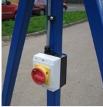
Isolator mounted on mobile gantry leg
